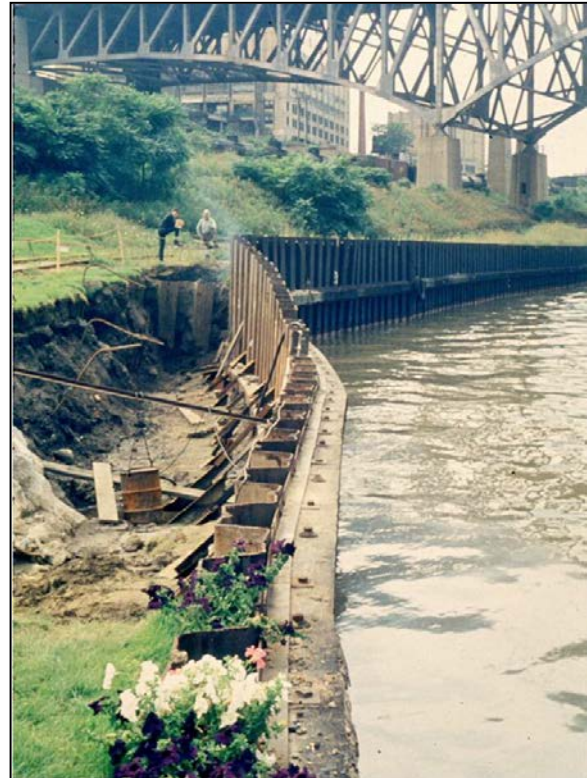
Figure 8-30 Sheet Pile Wall Failure
