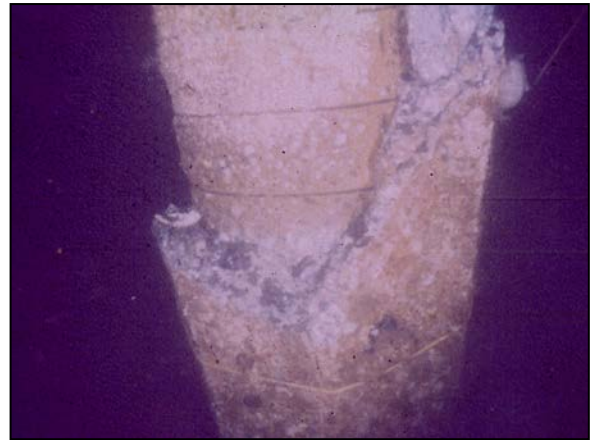
Figure 3-7 Failed Precast Prestressed Pile Due to Delayed Ettringite Formation
