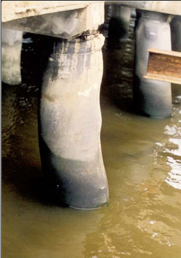
Figure 8-25 Displaced Fabric Formed Pile Jacket Due to Lack of Spacers and Uneven Grout Placement
