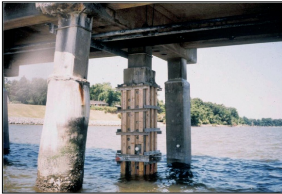
Figure 8-22 Completed Composite Jacket (Back Pile) and Jacket Read to be Pumped (Middle Pile). The Stiffening System is in Place on the Middle Pile Due to the Flexibility of the Fiberglass Jacket Form.
