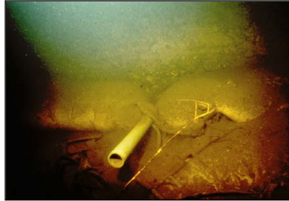
Figure 7-10 Grout Bag and Inlet Pipe
