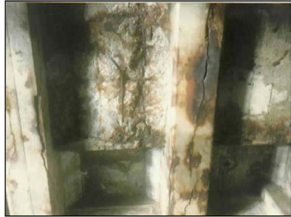
Figure 3-6 Cracks Along Reinforcing Bars
