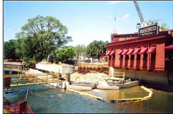
Figure 5-8 Bridge Pier with Dike Constructed of Soil, Traffic Barriers, and an Impervious Membrane
