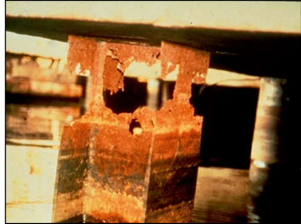
Figure 3-1 Steel Deterioration Resulting from Corrosion
