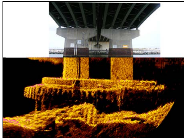
Figure 3-4 Undermining of Footings
